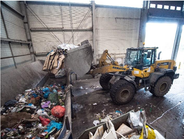
Photo 3: Front-end loaders pick up the mixed municipal waste and take it to a conveyor system which feeds the new pre-shredder.
