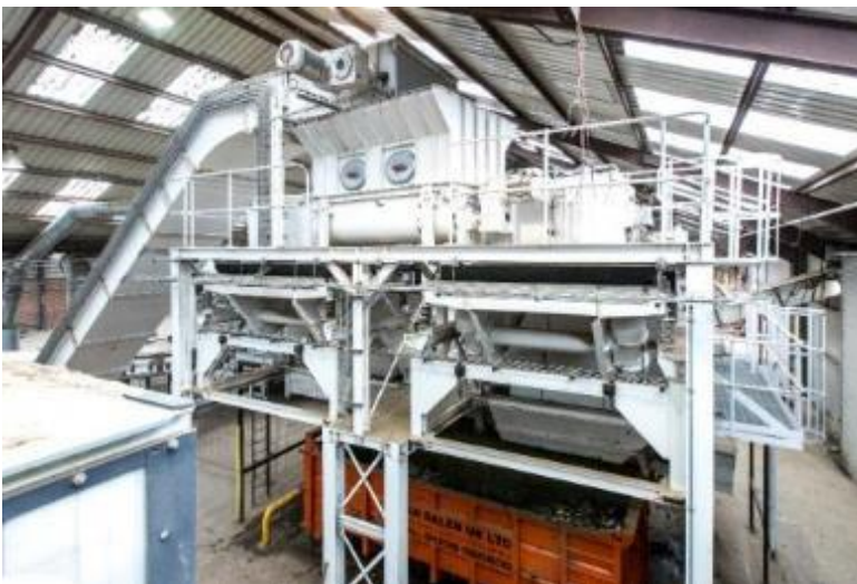
Photo 4: Non-ferrous metals like aluminium, copper and brass are taken out further down line by eddy-current separators.
